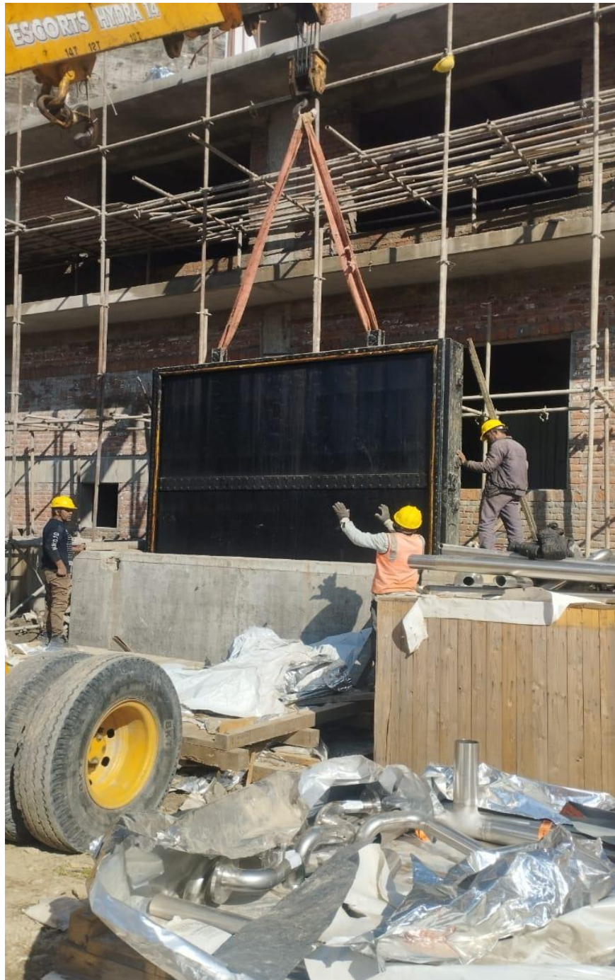
Dry Testing of Turbine Outlet Gate
