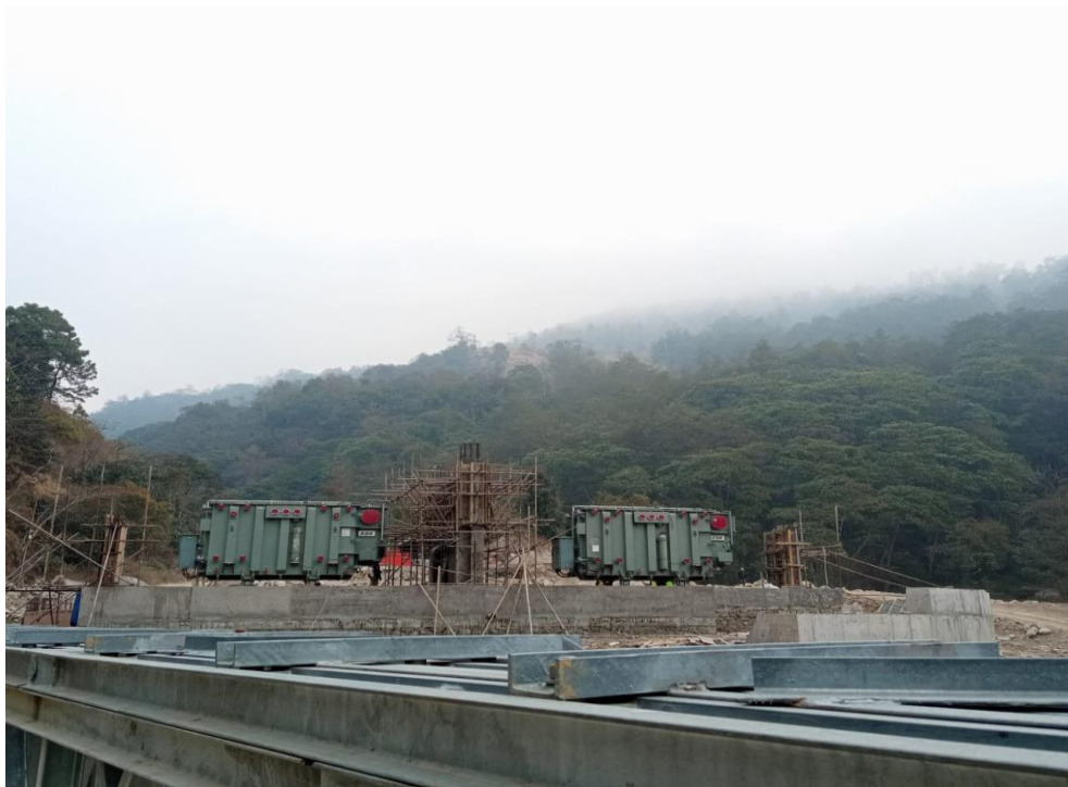
Transformer yard and transformer
